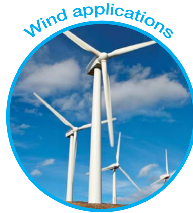
NH fuse links can be found in a wind turbine
