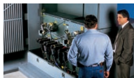
COOPER Power Systems
