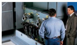
COOPER Power Systems
